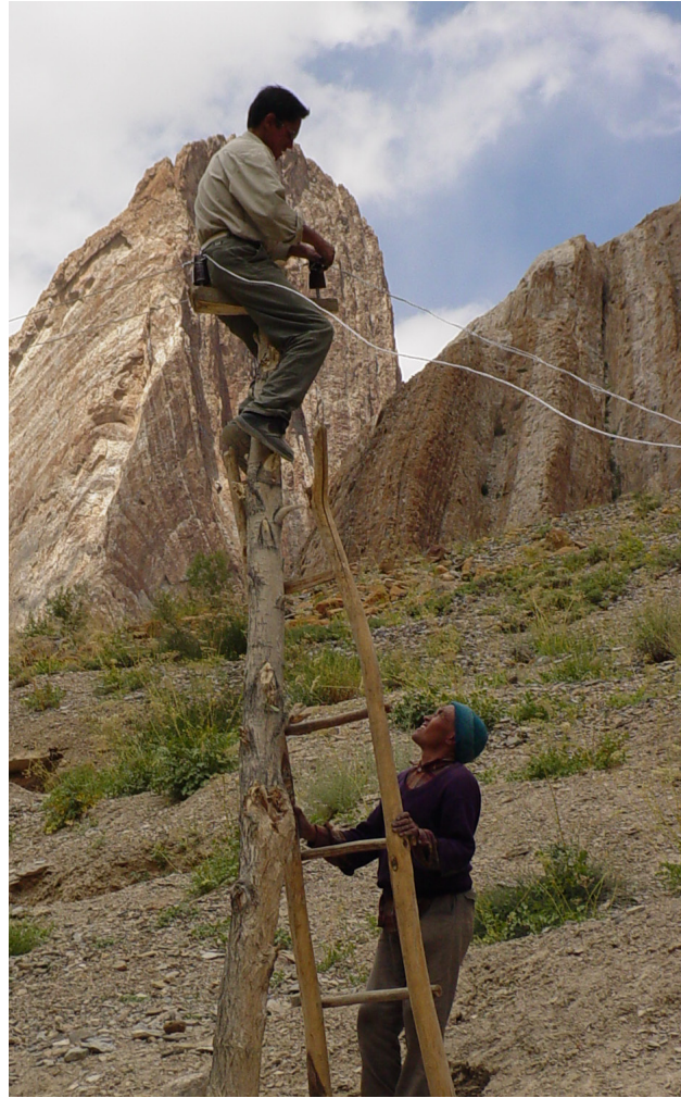
Micro-hydro transmission line being installed by the Ladakh Ecological Development Group (LEDeG) with Honupatta villager in Ladakh, India. Photo by Dipti Vaghela.
